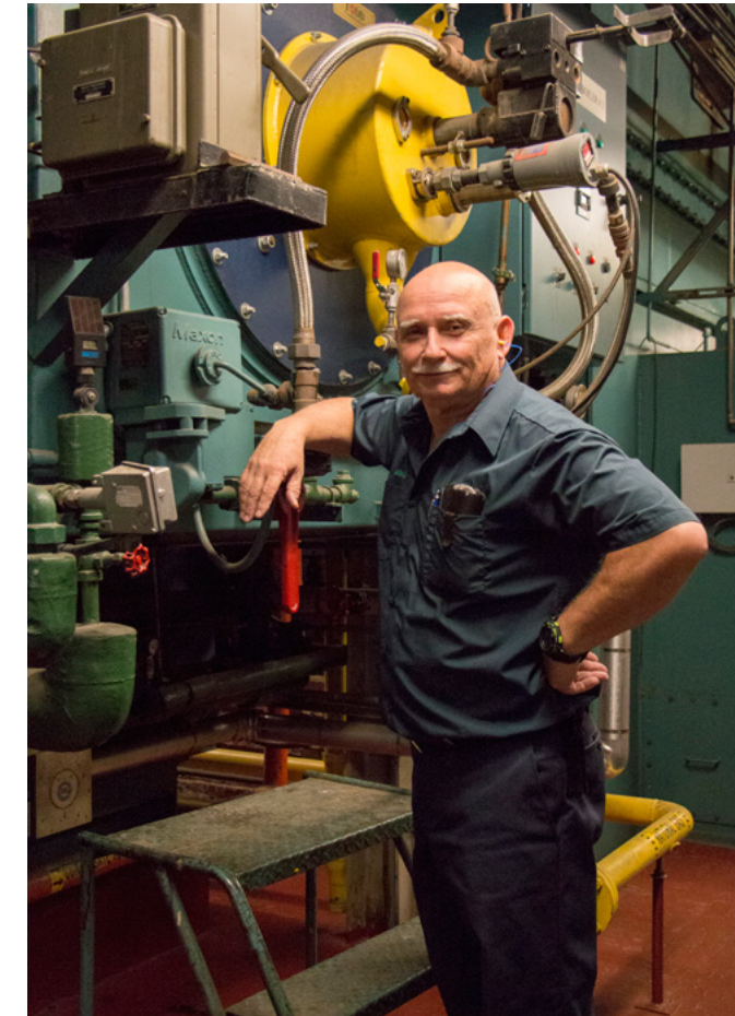
Above: Meet member Mike Gillis, of Local 119. Mike is a Power Engineer who's been working at the Nova Scotia Central Heating Plant for the past 28 years. He operates 4 boilers that provide heat and air conditioning to the Dartmouth General Hospital, Laundry Services, NSCC Waterfront Campus, and The Nova Scotia Hospital.
